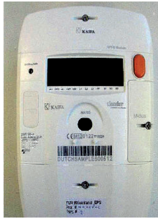
Slimme meter KAIFA DSMR4.0. GPRS transmissie
